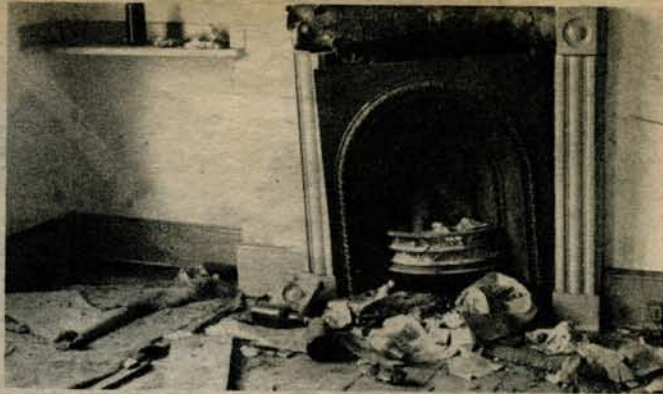
An internal view of the second floor of 213 North Gower Street — before the squatters moved in. At this time the basement was open to the sky through holes in roofs, ceilings and floors. The windows were broken and basins and lavatories had been smashed.
