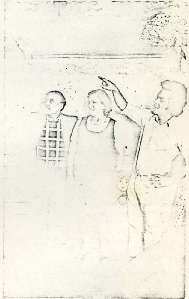
● Mr Anthony Piery (right) interprets the despair of his mother and father in law Mr and Mrs Mell, and shows the damage caused by years of a leaking roof.
